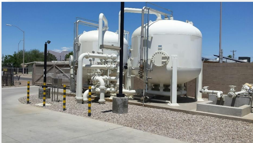
Figure 8 – GAC Treatment (Flowing Wells Irrigation District)
